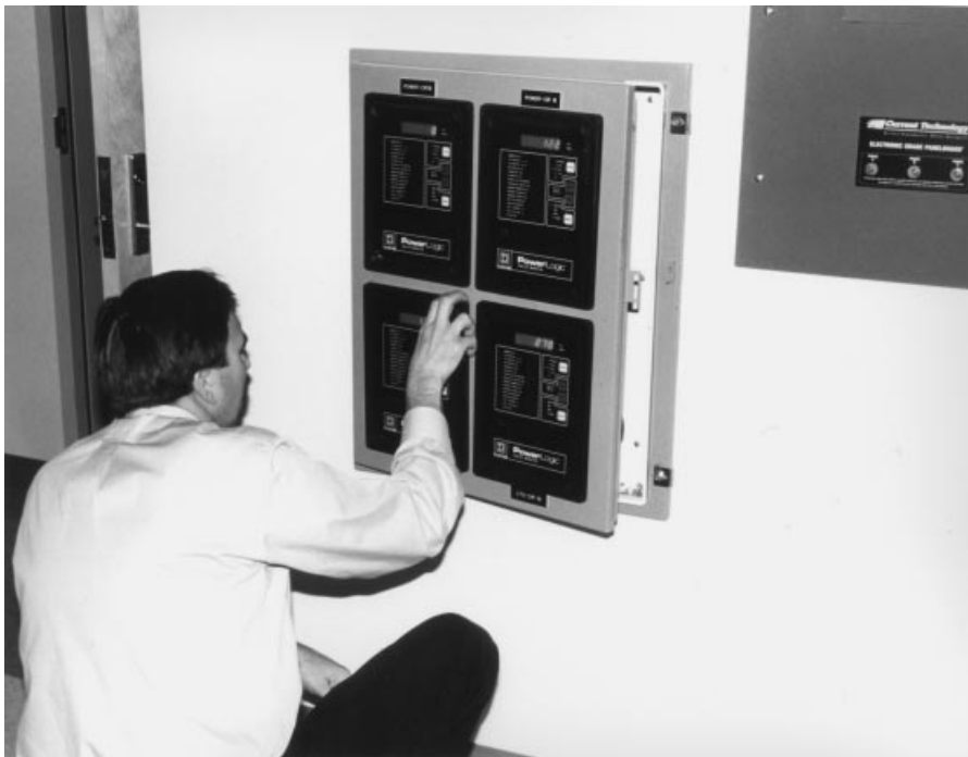
Fig. 7. More than 280 sensors integrated into the ITL Laboratory monitor its pulse, such as the electrical system.
